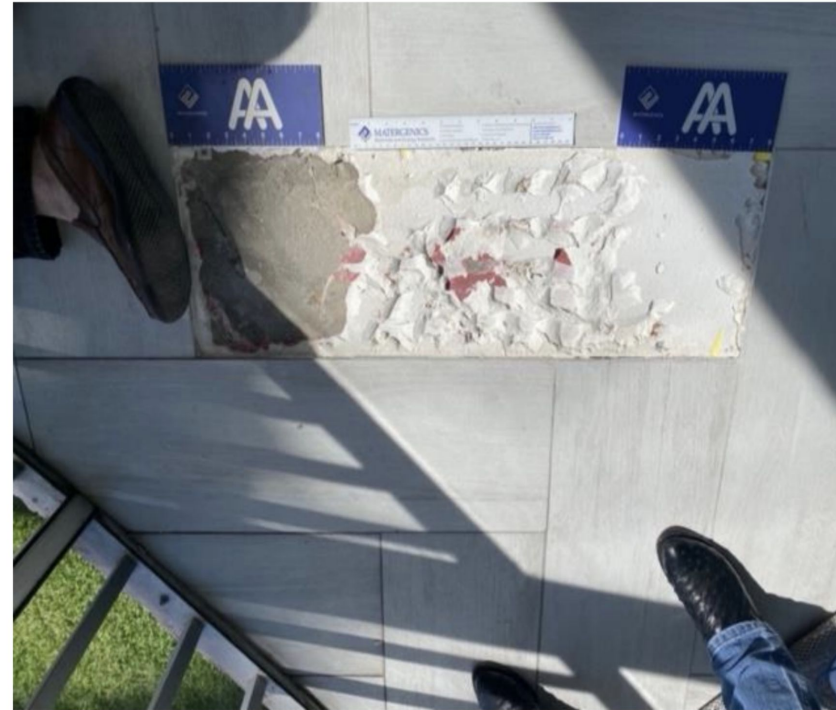
Area selected for corrosion risk assessment exhibiting mortar and water proofing coating
